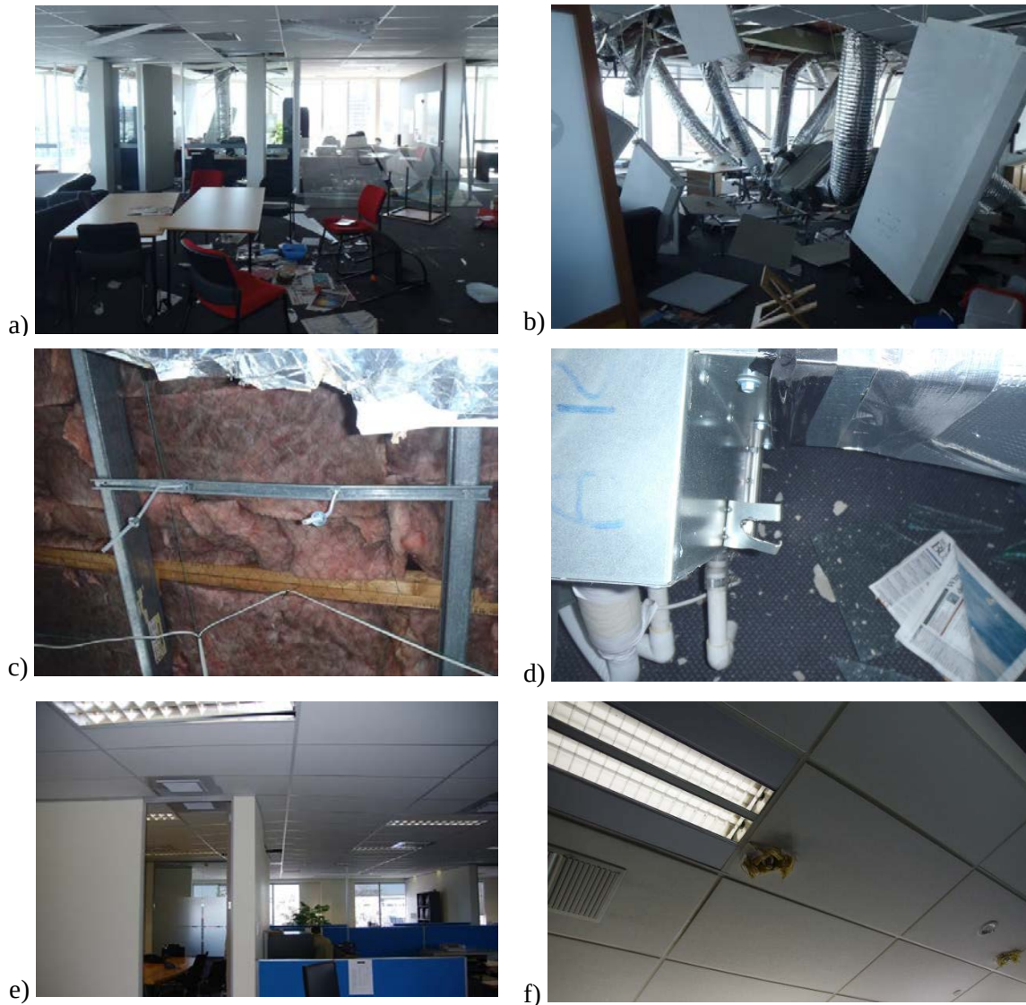
Figure 2. Observed damage to overhead NSEs following the Canterbury Earthquakes; a) dislodged ceiling tiles and glass partition, b) HVAC unit fallen through ceiling, c) HVAC supports failed, d) failure of HVAC unit fixing, e) distortion of ceiling grid from wall, f) damage to ceiling tiles around sprinkler heads.
